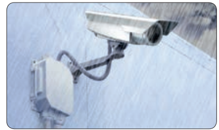
Installation with free cables.
